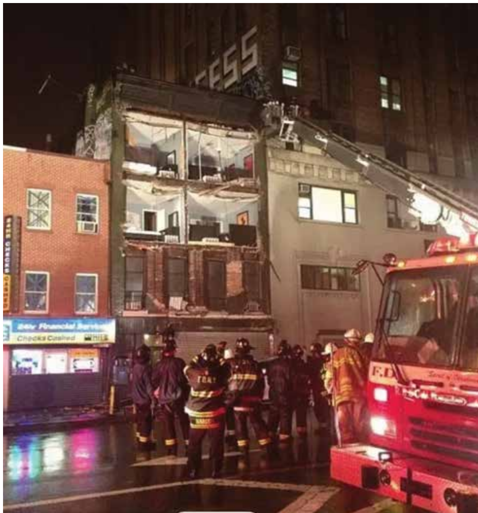
92 EIGHTH AVENUE , center, was a victim of Hurricane Sandy in 2012. Its front façade, above the second floor windows, collapsed in the night exposing the illegal interiors. Credit: 6sqft NYC.
