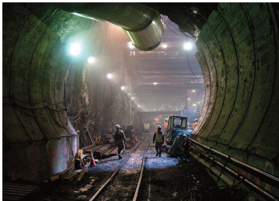
TWO TRADESMEN WALKING INTO THE LAUNCH BOX from the west side tunnel. The tunnel is twenty two feet in diameter, 1/21/2011.
